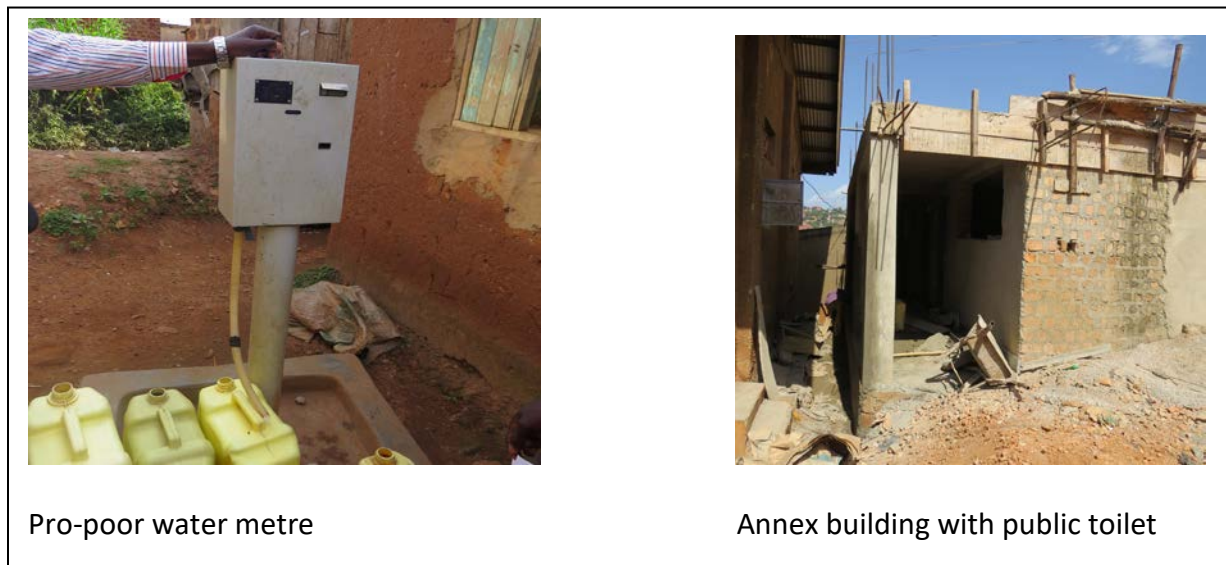
Figure 1: Pro-poor water metre in Luzira ward and community centre annex building with accessible toilets under construction at Banda
